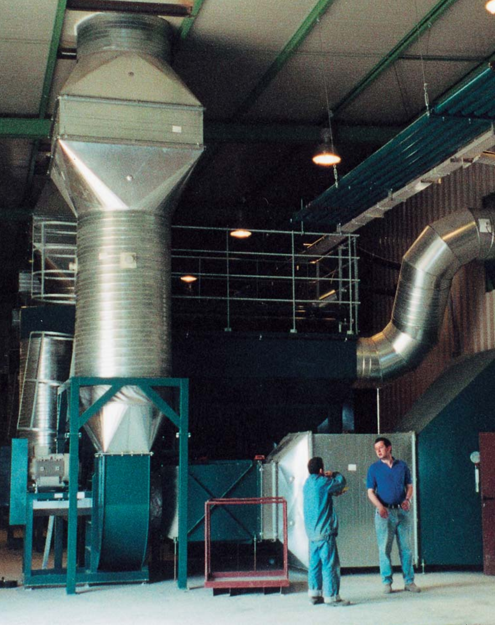
Combined dust and paint exhaust system seen from machine room side
