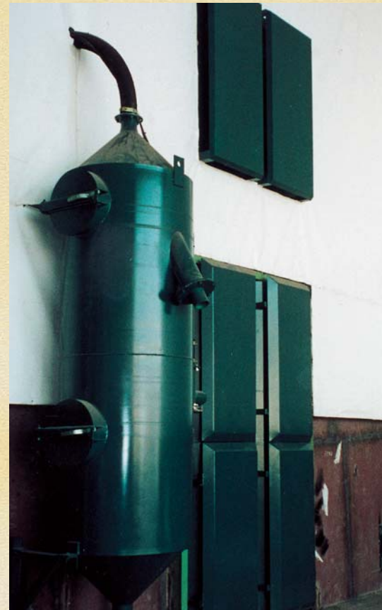
Exhaust labyrinths for respectively dust from blasting and from painting (upper & lower)
